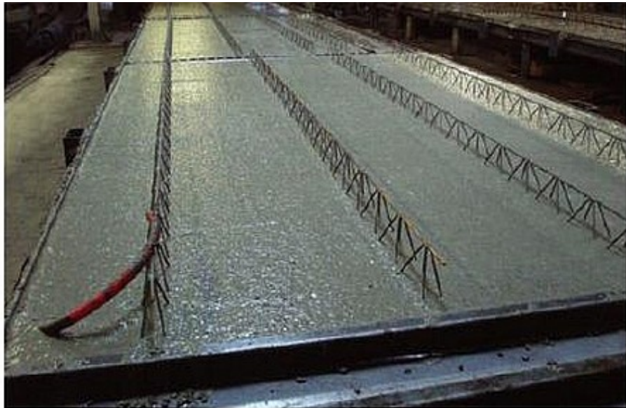
Concreted thermo-active floor element
