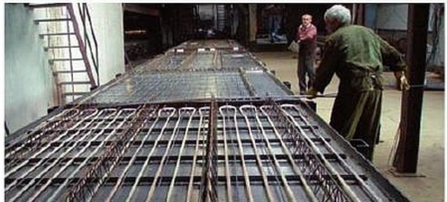
Once the pipe grid has been positioned in the pallet, the reinforcement is inserted
